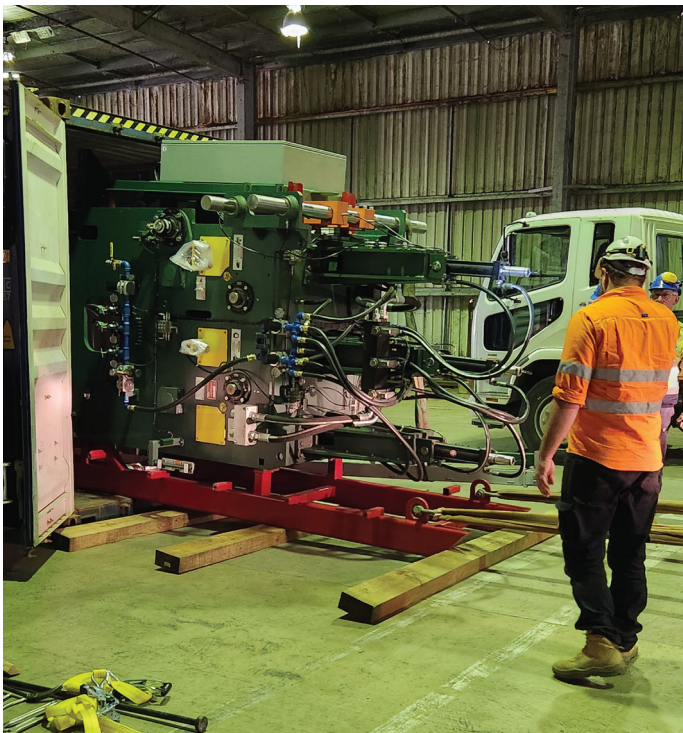
One of the seven containers of the HSS that has arrived.
