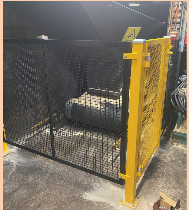
Guarding of conveyor tail drum nip point
