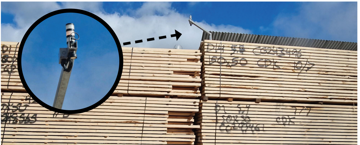
Over-height alarms now in operations.
