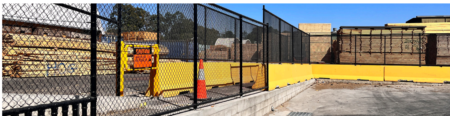
CDK Infeed Area's newly installed fencing for separation between pedestrians and forklift.
